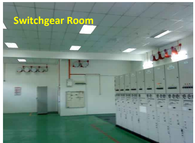
Tenaga Nasional Berhad (TNB) Malaysia, 2009
